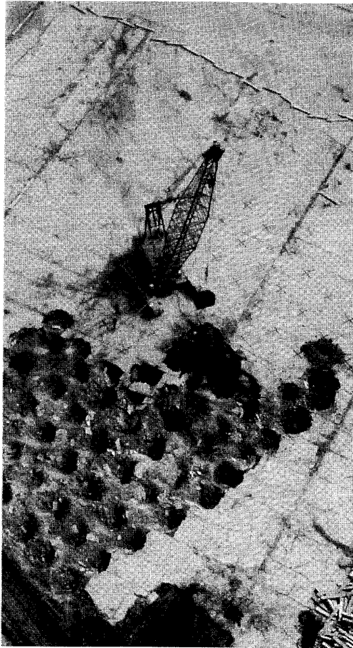
Figure 12.3 Aerial view of site undergoing soil improvement by dynamic compaction. The grid pattern on which the dynamic compaction weight is dropped, and the need for subsequent regrading and surface compaction, are evident from this photograph. (Photo courtesy of Hayward Baker).
